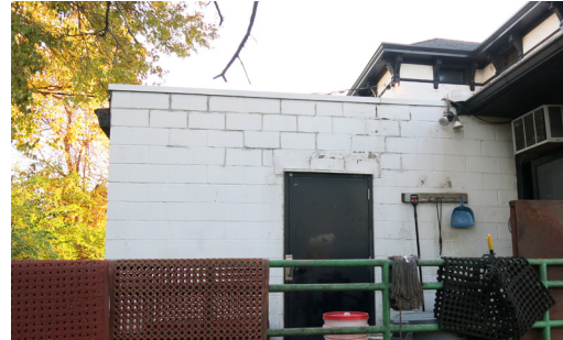
The non-historic kitchen addition is in fair to poor condition.
