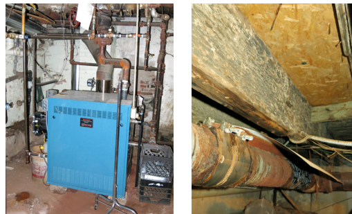
While the boiler itself is relatively new, it connects to deteriorated steam piping with many leaks and old patches.
