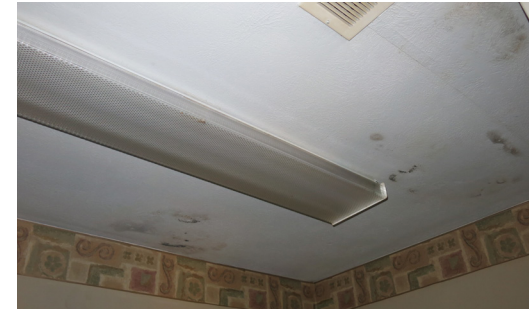
Minor damage to restroom ceiling in non-historic addition.
