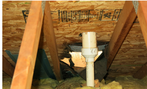
Hole in roof of non-historic vestibule addition caused by falling tree. This has been temporarily covered with a tarp but continues to leak.
