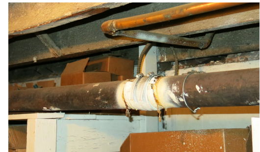
Patch at leak in deteriorated steam pipe.
