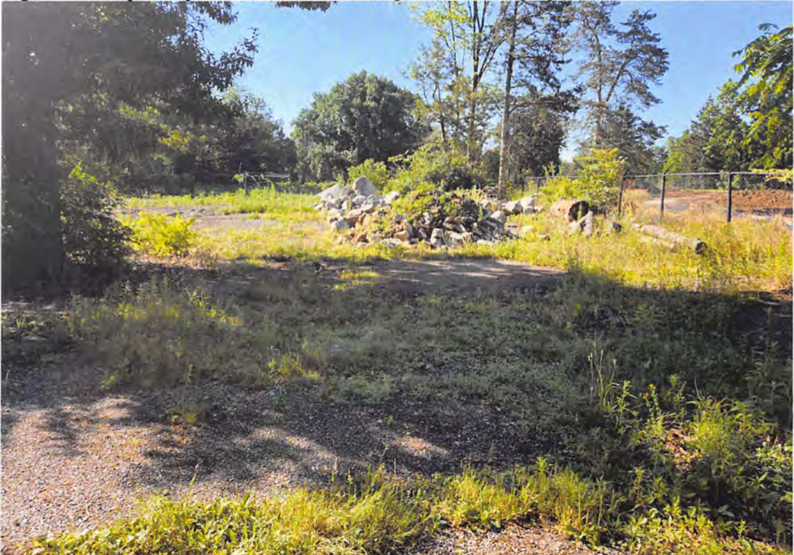
Figure 15. More waste piles of construction materials within the project.
