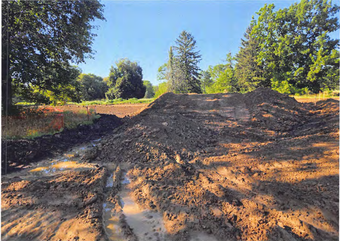
Figure 10. Spoil piles and grading activity in the southern portion of the project.
